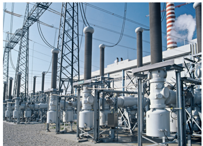
Fig. 2/8 Application in the high-voltage system
